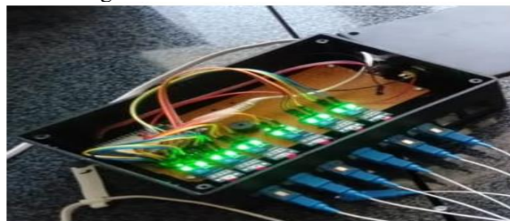
Figure 17. Condition of All ODC Cables Installed
